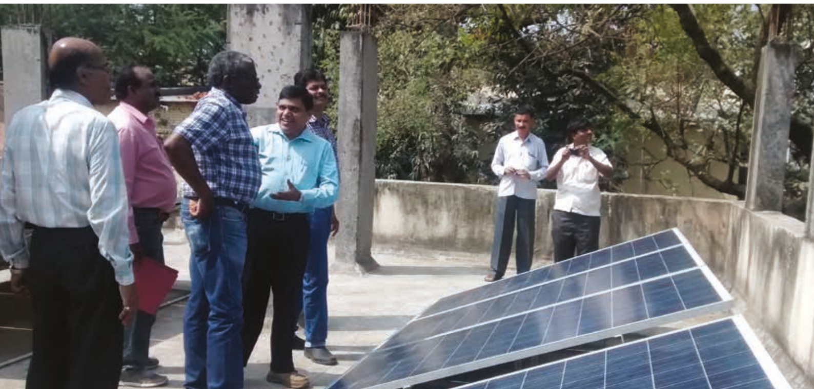
Model solar panel installation at a PHC in Maharashtra
