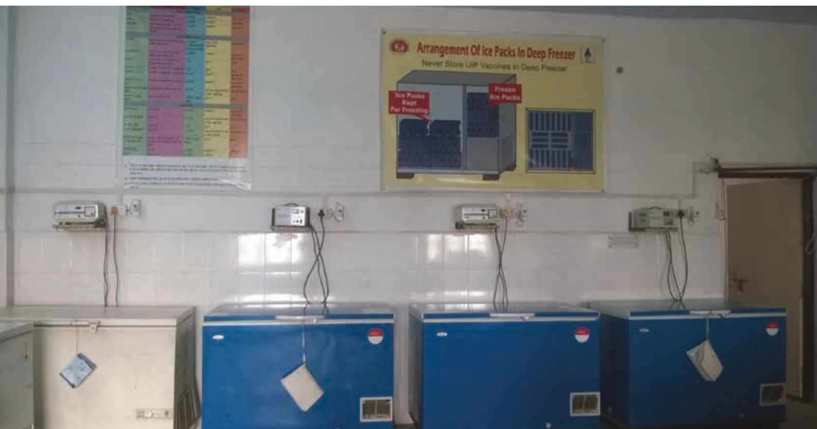
A well maintained cold chain room in a health facility
